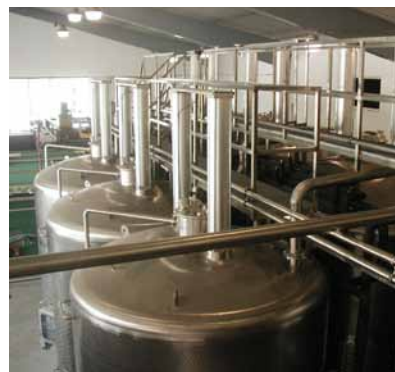
Dosing tanks and reservoirs
